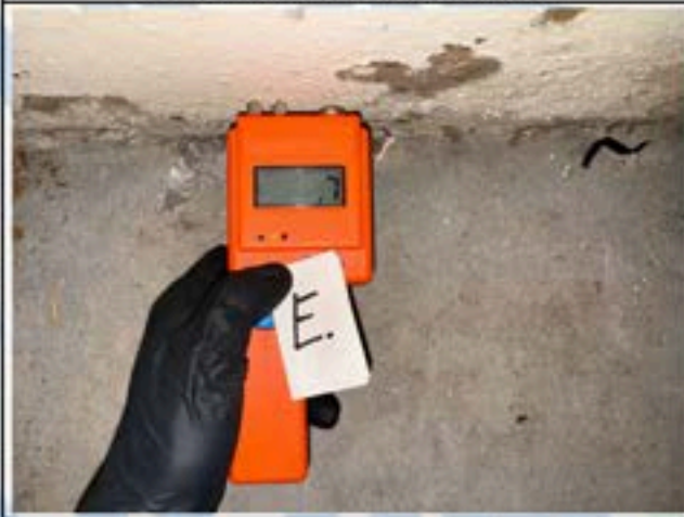
Kitchen Elevated Moisture Content
