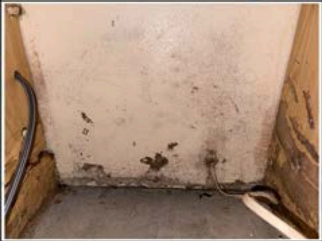
Kitchen Visible Suspected Growth
