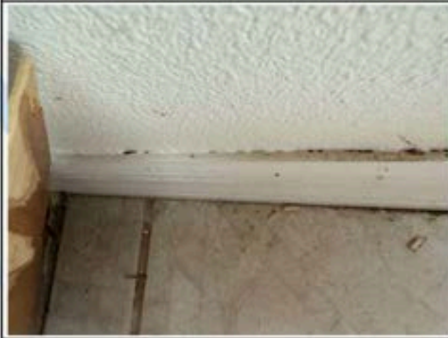
Dining Room Visible Water Damage
