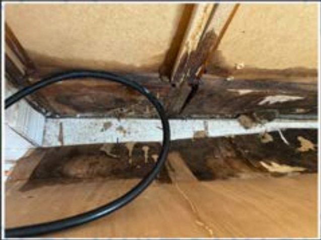
Dining Room Visible Suspected Growth
