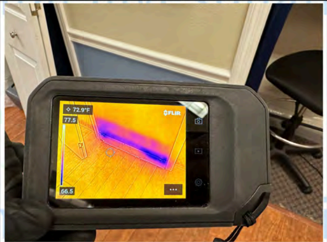
Main Hall 4 - Thermal Imaging
