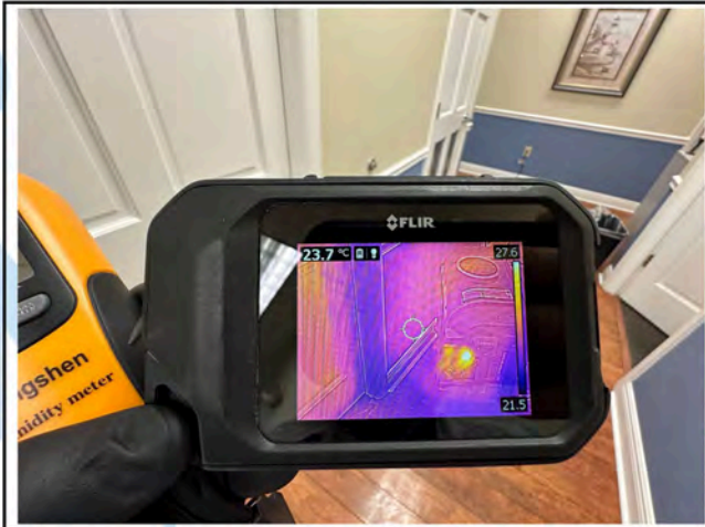
Main Hall 2 - Thermal Imaging
