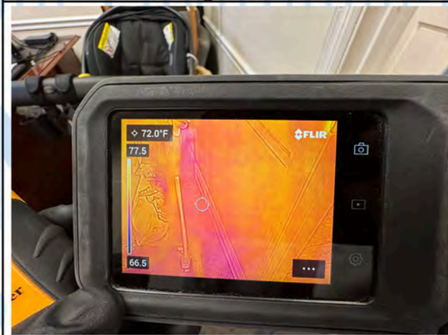
Manager's Office - Thermal Imaging
