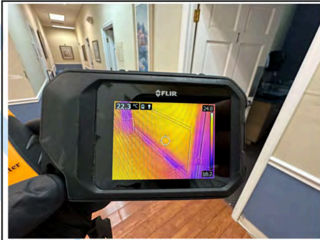
Main Hall 2 - Thermal Imaging
