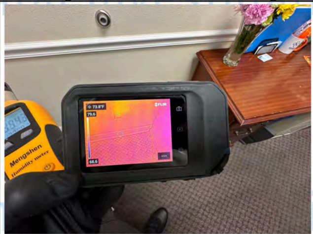
Manager's Office - Thermal Imaging
