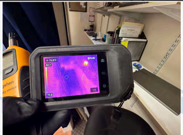
Main Hall 4 - Thermal Imaging
