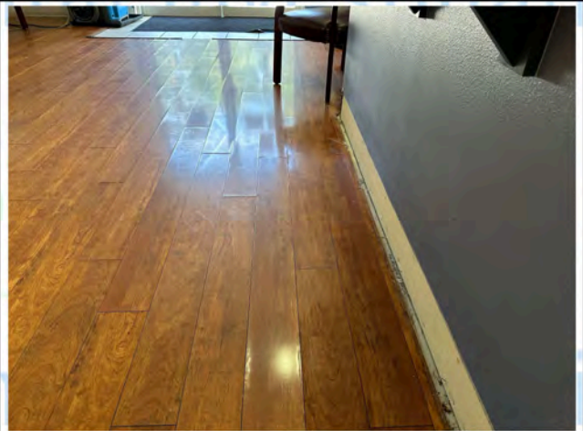
Waiting Room - Visible Water Damage
