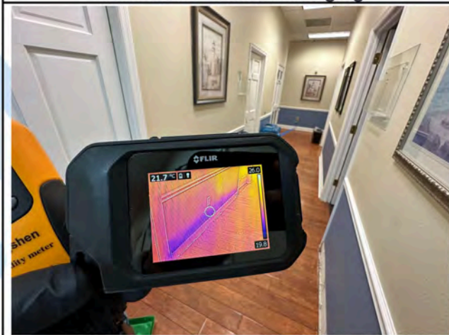
Main Hall 2 - Thermal Imaging
