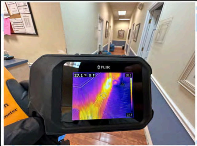
Main Hall 2 - Thermal Imaging
