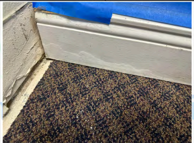
Room 1 - Visible Water Damage
