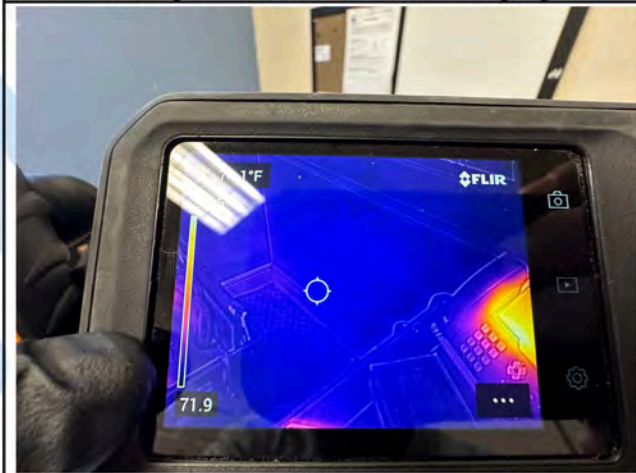
Manager's Office - Thermal Imaging
