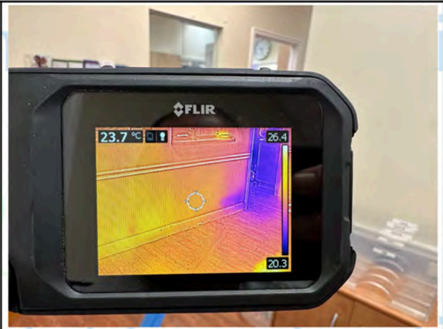
Main Hall 1 - Thermal Imaging
