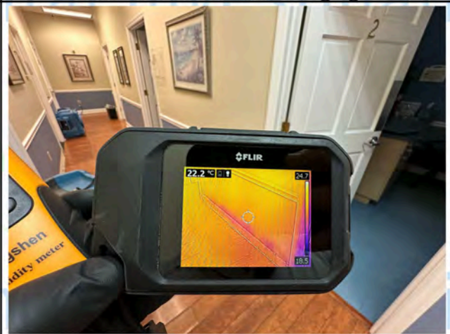
Main Hall 2 - Thermal Imaging
