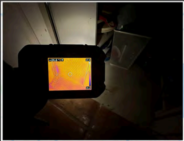
Dining Room Thermal Imaging
