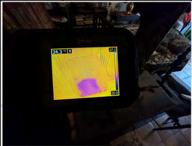
Dining Room Thermal Imaging
