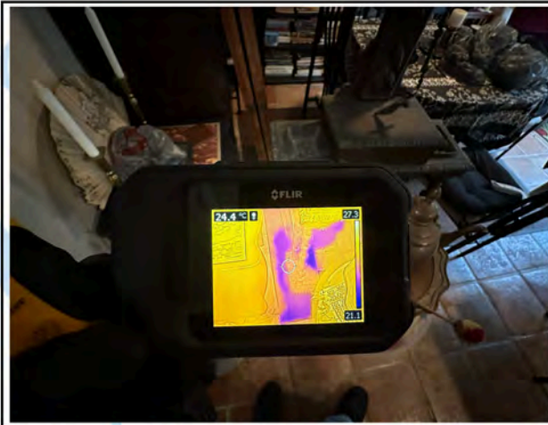
Dining Room Thermal Imaging
