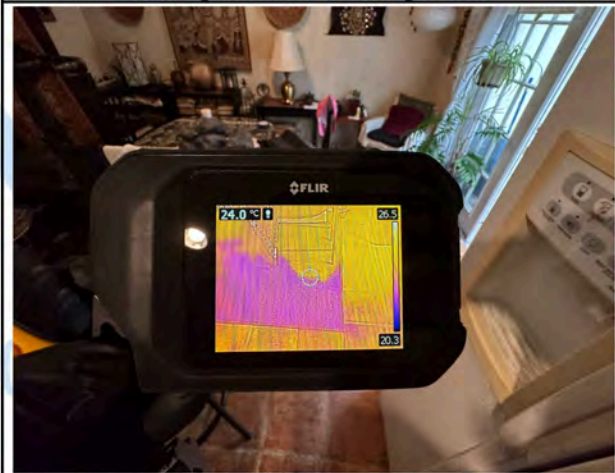
Dining Room Thermal Imaging
