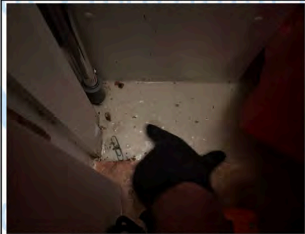
Dining Room Standing Water
